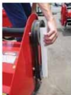
Check the vertical alignment of the pulleys using a spirit level. The pulleys must be absolutely parallel.
